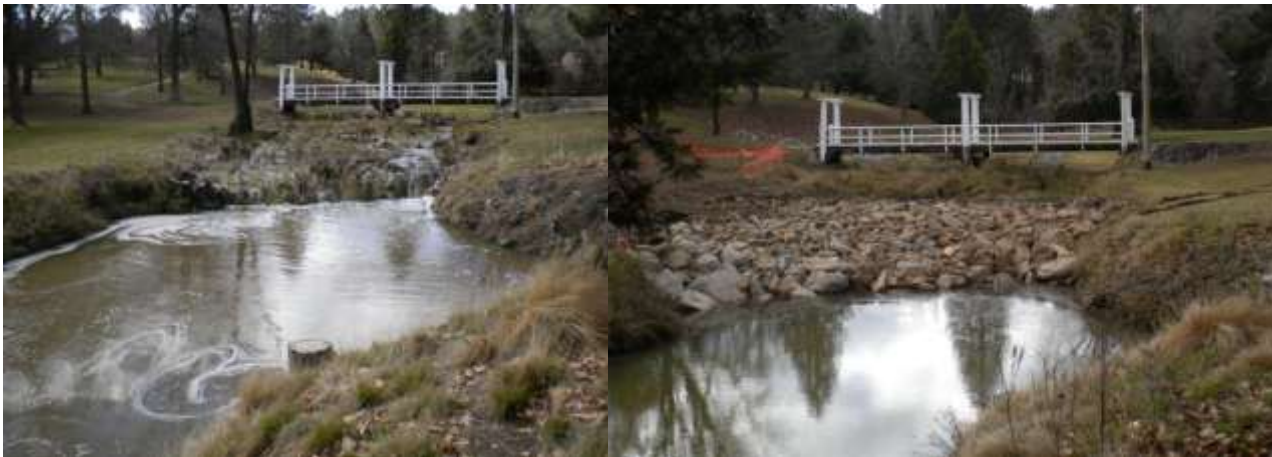
Alma Park footbridge showing severe head cut in Rocky Creek on left and rock ramp remediation work on right.
